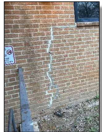
View of cracks in Brick Veneer
