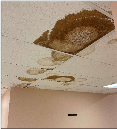
Views of water leaks above the ceiling
