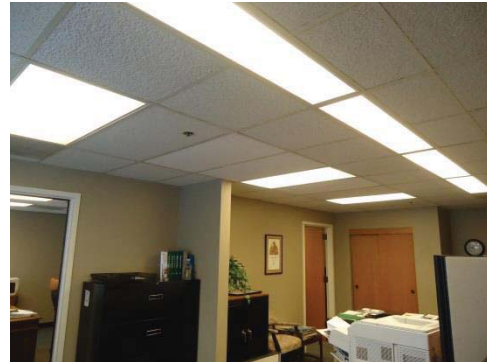
Photo 4 - Existing Lighting Fixture
