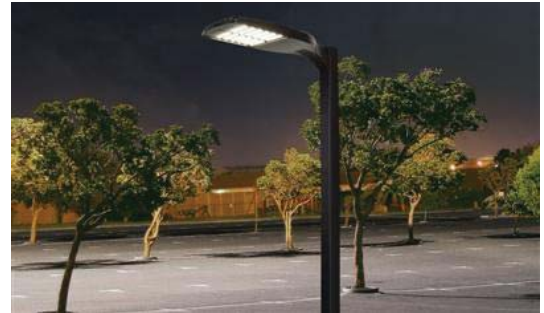
Photo 6 - Typical LED Fixture
