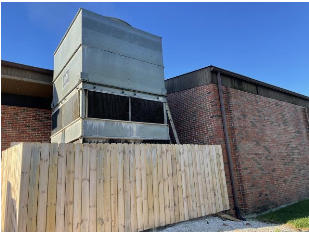
Photo 3 – Existing evaporative condenser
