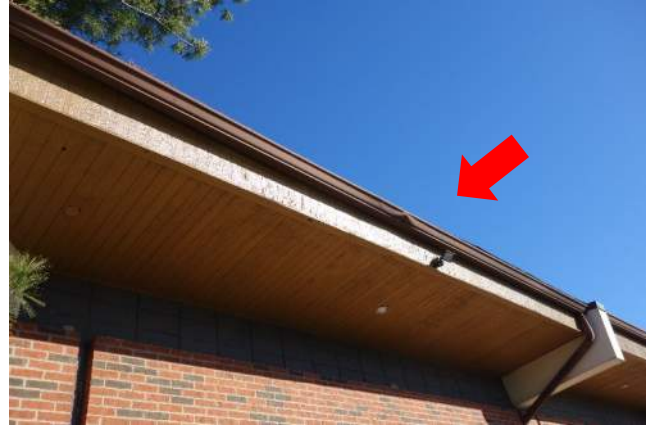
Figure 10 – Damaged Gutter Sections
