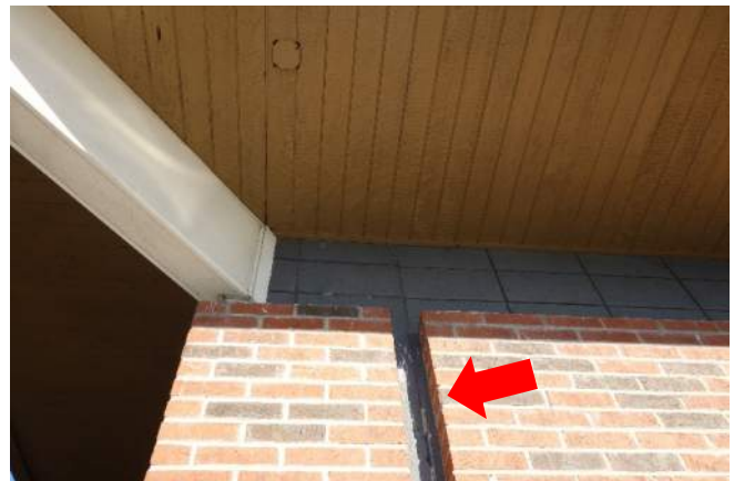
Figure 12 – Vertical Masonry Joint Crack
