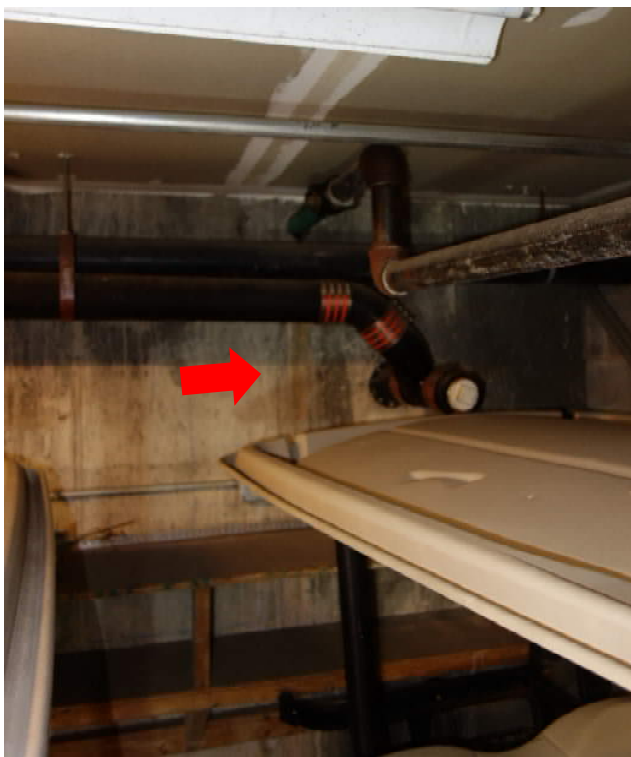
Figure 24 – Vertical Hairline Crack
