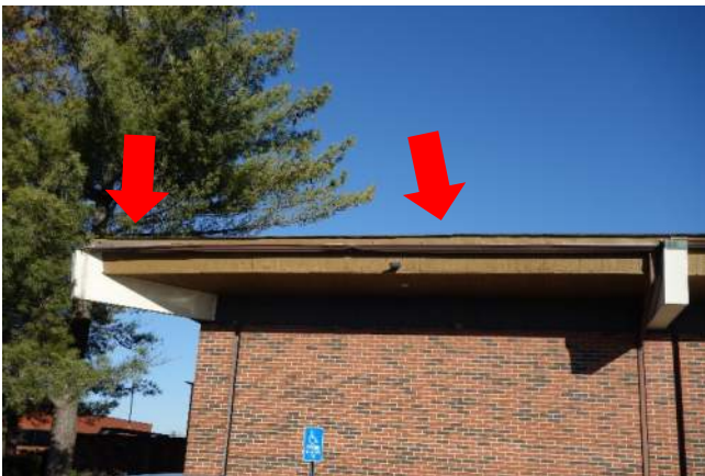
Figure 11 – Damaged Gutter Sections
