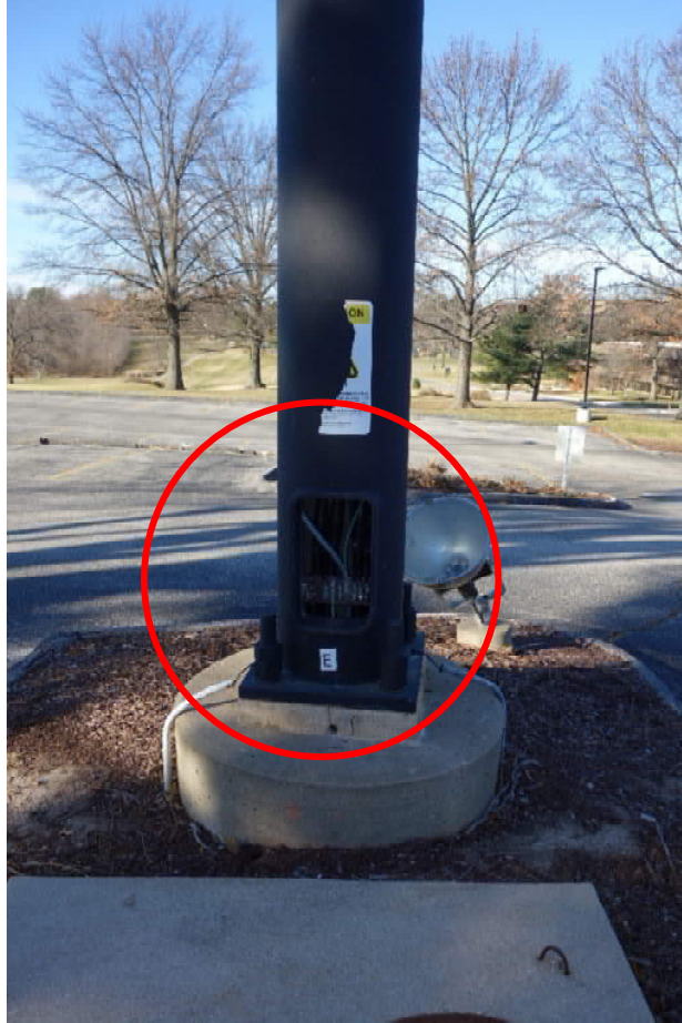
Figure 32 – Missing Cover Plate to Light Pole
