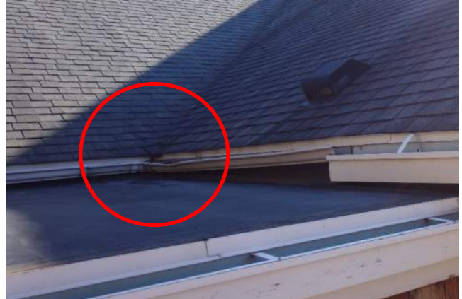
Figure 5 – Gutter Damage Above Offices
