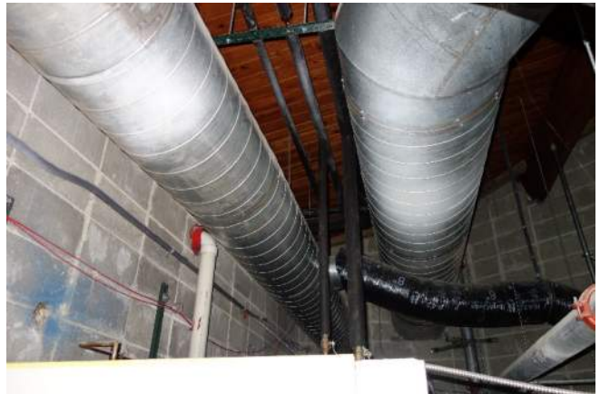
Figure 21 – Mechanical Area above Bathrooms
