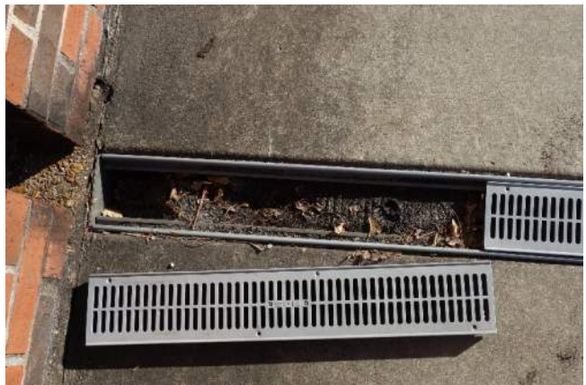
Figure 7 – Sediment Filled Drainage Channel
