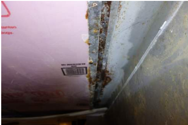
Figure 26 – Rust under Ceiling Drywall
