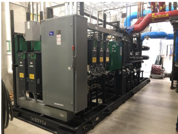
Photo 11 - Example of an Indirect CO 2 Chiller Package
