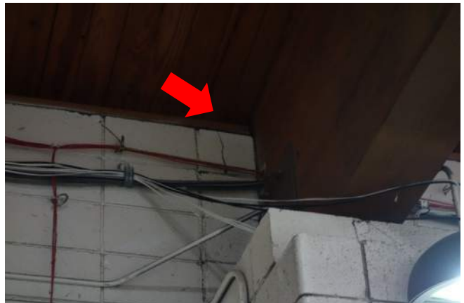
Figure 23 – Crack in Masonry Block
