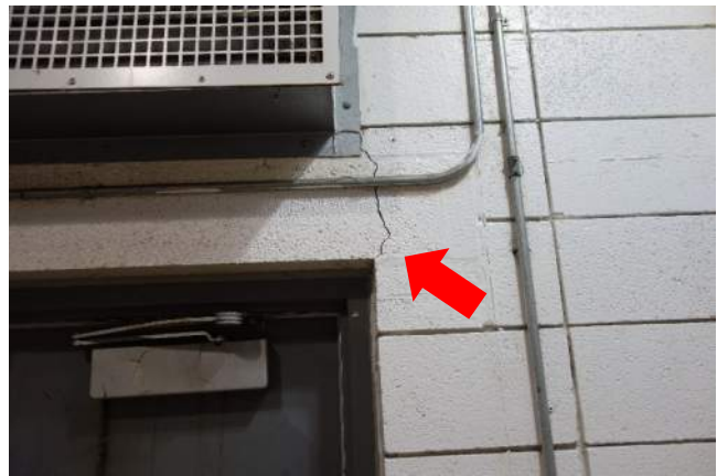
Figure 19 – Concrete Header Beam Crack
