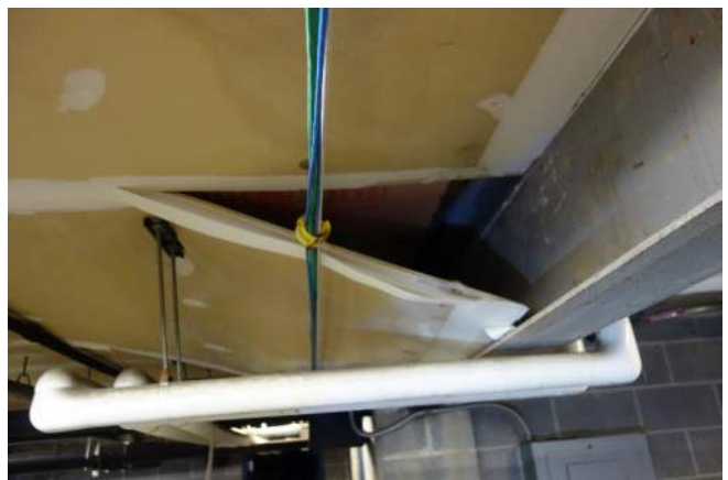
Figure 25 – Falling Ceiling Drywall
