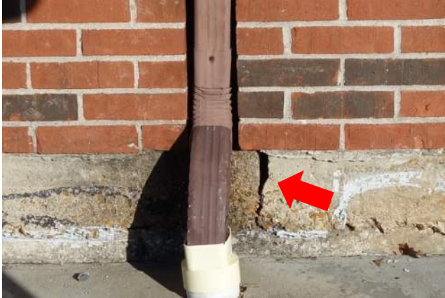
Figure 9 – Foundation Joint Separation
