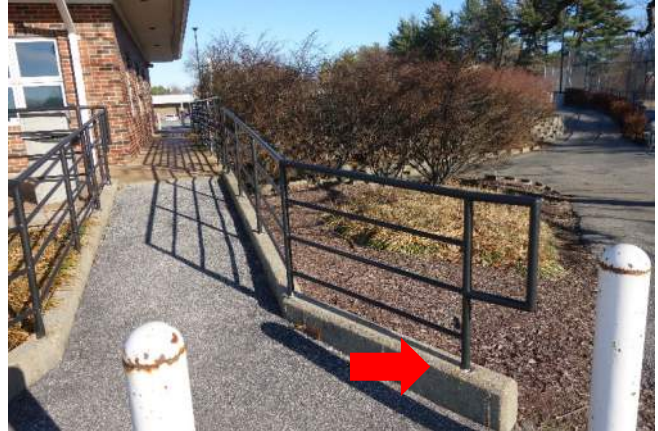
Figure 16 – Loose Railing Section
