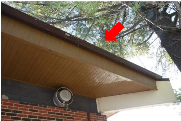
Figure 13 – Damaged Gutter Sections
