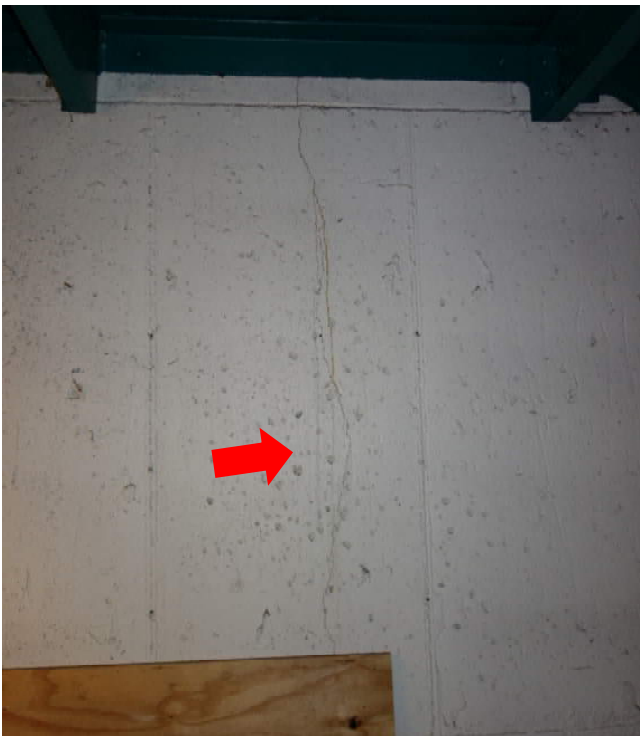
Figure 30 – Vertical Hairline Crack
