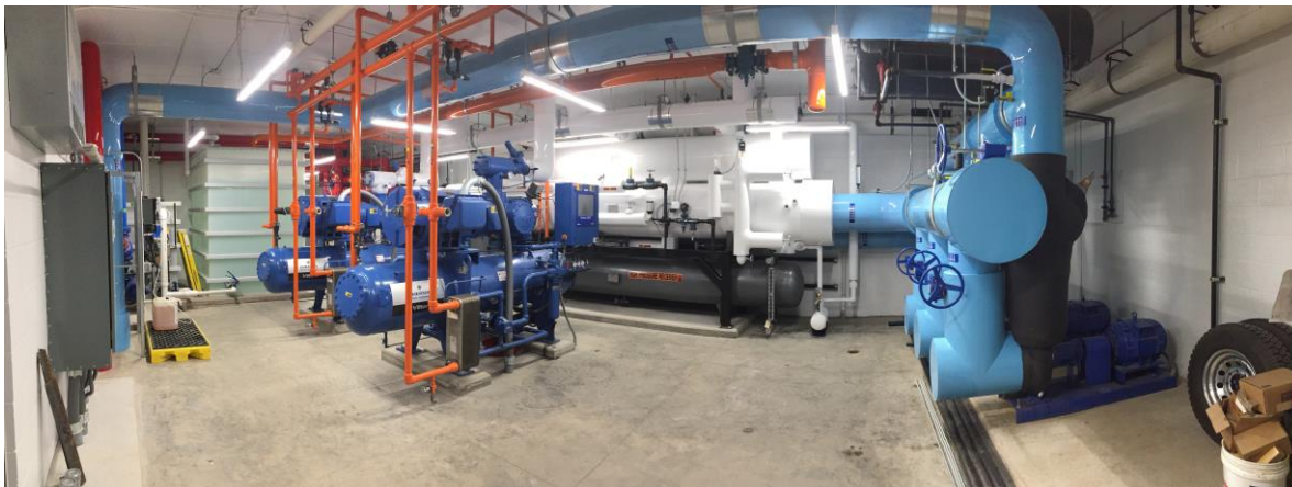
Photo 10 - Example of a stick-built industrial grade, flooded ammonia-based system
