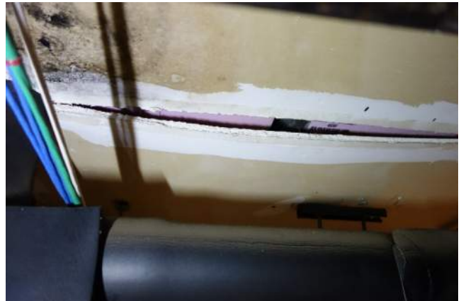
Figure 27 – Falling Ceiling Drywall
