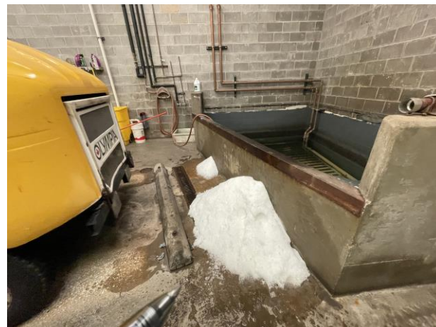
Photo 4 – Existing snow melt pit and coil
