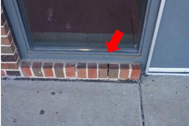
Figure 4 – Mortar Joint Damage
