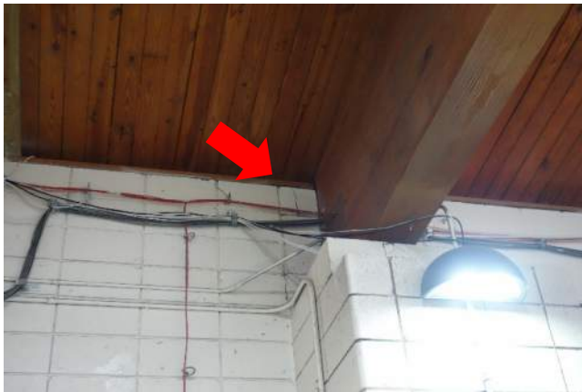
Figure 22 – Crack in Masonry Block
