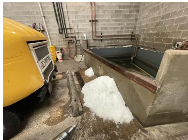
Photo 4 – Existing snow melt pit and coil
