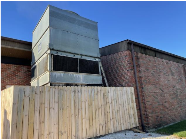
Photo 3 – Existing evaporative condenser
