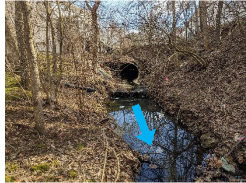
Figure 6-16: Knickpoint at outfall
