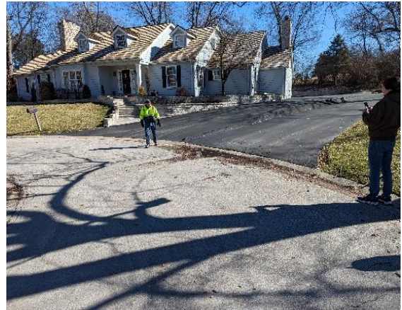
Pooling at end of driveway
