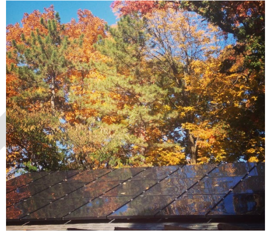
Rooftop solar array on home in Creve Coeur
