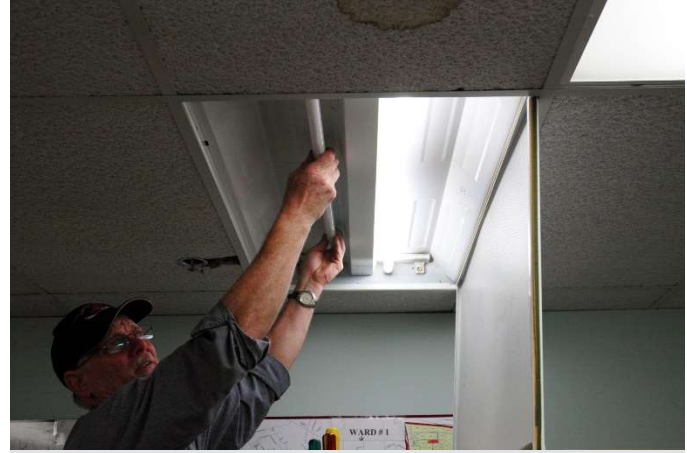
Lighting at all municipal facilities has been retrofit with energy efficient fixtures.
