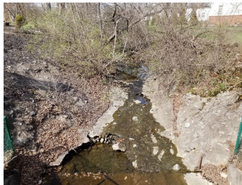
Failing grouted riprap
