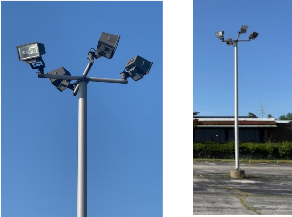
Figure 8: Existing parking lot lighting to be angled down.
