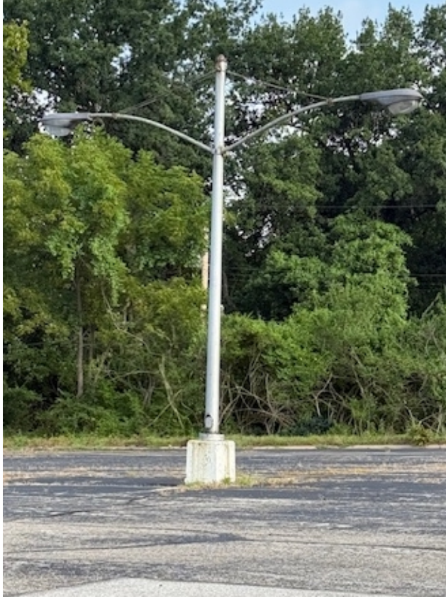
Figure 2. Example of non-conforming light poles being replaced.
