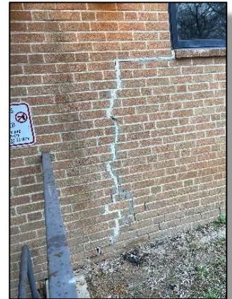
View of cracks in Brick Veneer
