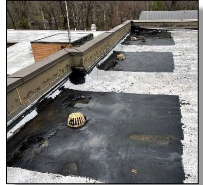
Existing roof condition were patched due to leaking.
