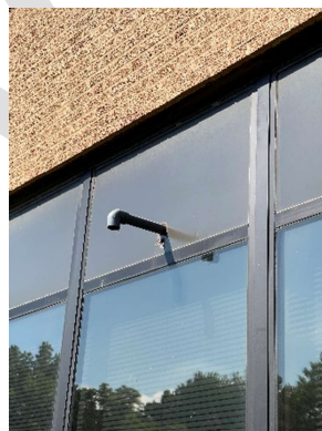
Condensation Drain out of window panel. No caulk around pipe / water & insect infiltration
