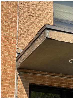
Peeling paint and deteriorating wood fascia on canopy
