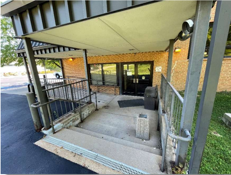
Existing Entry into Community Room – Despite drain at top of step and area drain at landing, entry doors are subject to flooding should area drain gets clogged or covered.
