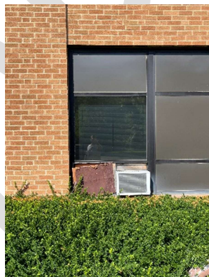
Plywood filler is falling out of window at air conditioner
