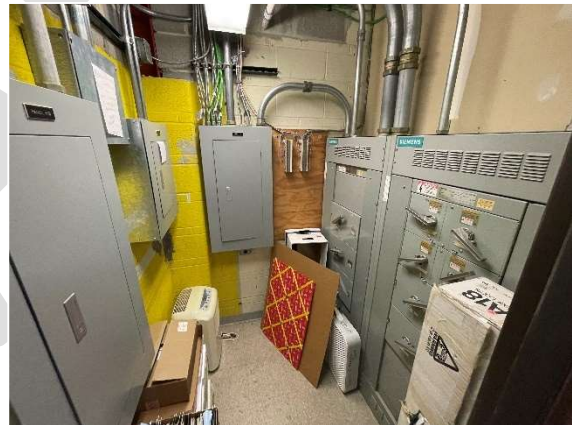
Electrical panels and switch gear is being blocked by storage items resulting in code violations.
