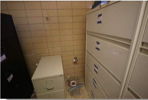
Old restroom was converted into file storage room. Existing infrastructure was left in place.
