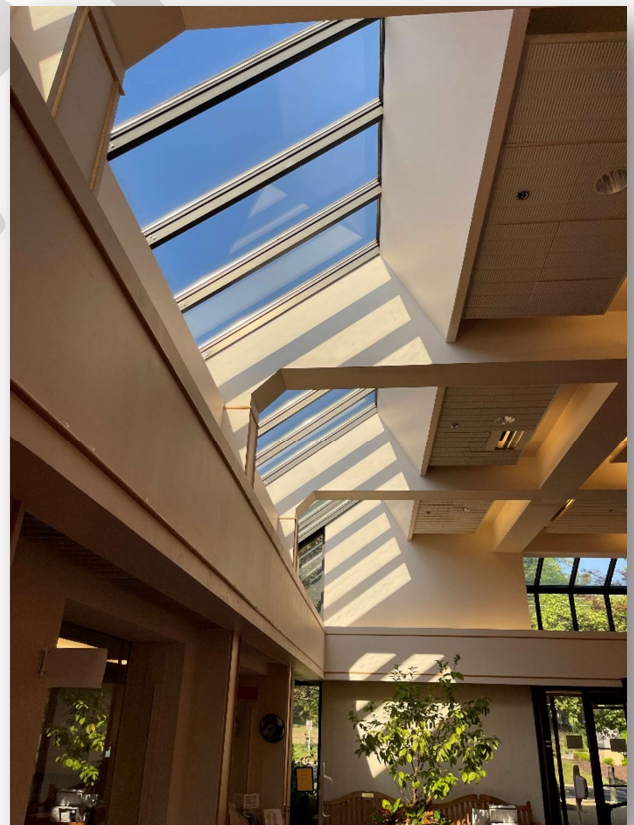
View of Existing Main Entrance Lobby / Skylights along South side of Lobby
