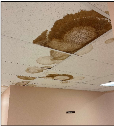
Views of water leaks above the ceiling
