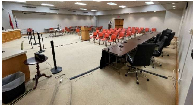
View of Council Chambers and wire raceways with wire and cables running on surface of floor being protected by tapered rubber covers.
