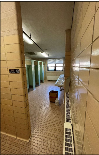
Existing Restroom with narrow passage and antiquated plumbing fixtures
