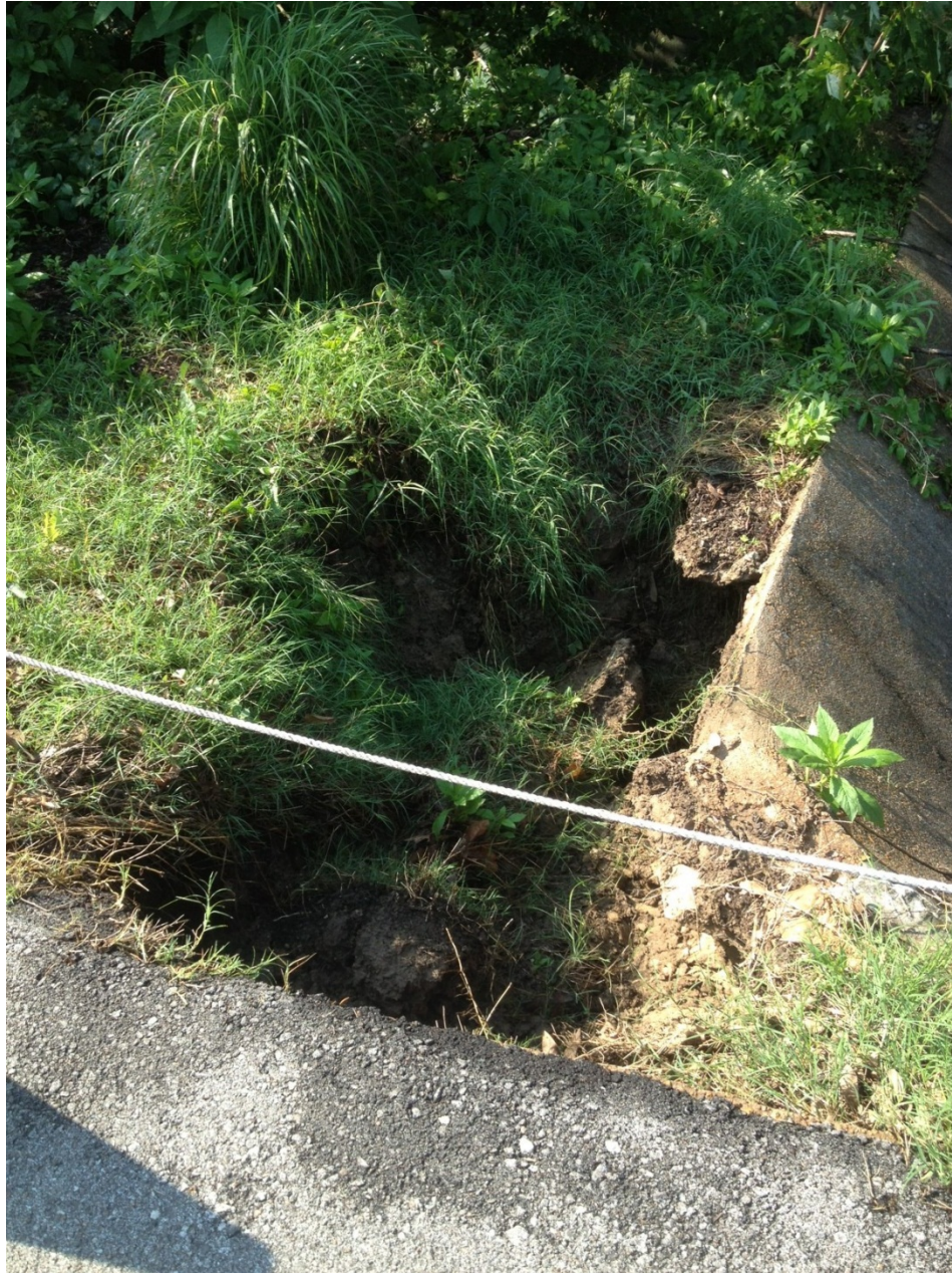
Photo 3: On top of the dam, looking south from the cart path. The June 17 storm re-opened the breach in the dam and exposed a significant hole in the dam. Water is using this route as its path. The concrete channel (i.e. where the water should be flowing) begins at the right side of the photo, and the side wall shown is completely undermined. The hole shown here is more than six feet deep and extends back under the cart path.
