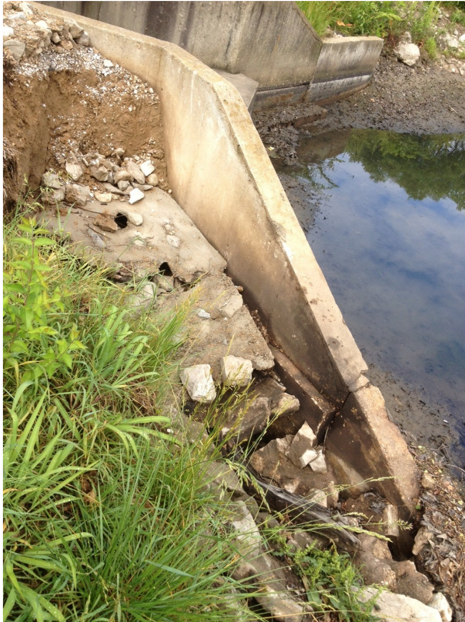
Photo 1: The initial breach of the dam occurred along the side of the spillway. (The spillway wall is the closest of the concrete walls shown here.) The top foot of the detention pond drained out through the breach, which began at the bottom right corner of the photo. Note the grouted rock lining of the dam is shown collapsed into the breach. It was apparently hollow underneath and hid the issue from view.
