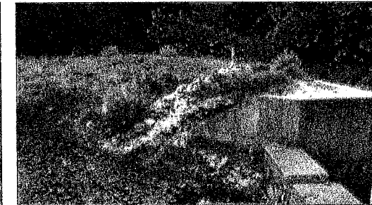
Piping through earthen dam at the existing overflow on Dielman Dam
