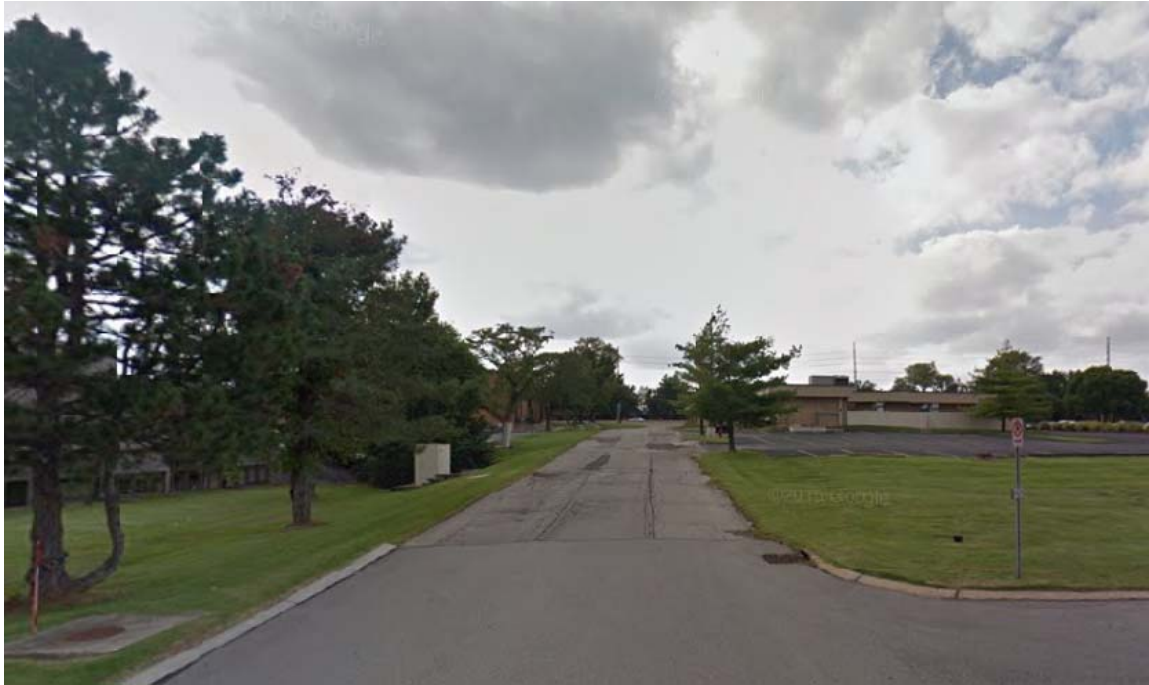
Figure 1: Google street view of Woodfield Lane looking west from the cul de sac of the City's portion of Woodfield. Note the clear pavement condition change from the public street (foreground) and the private street (background).
