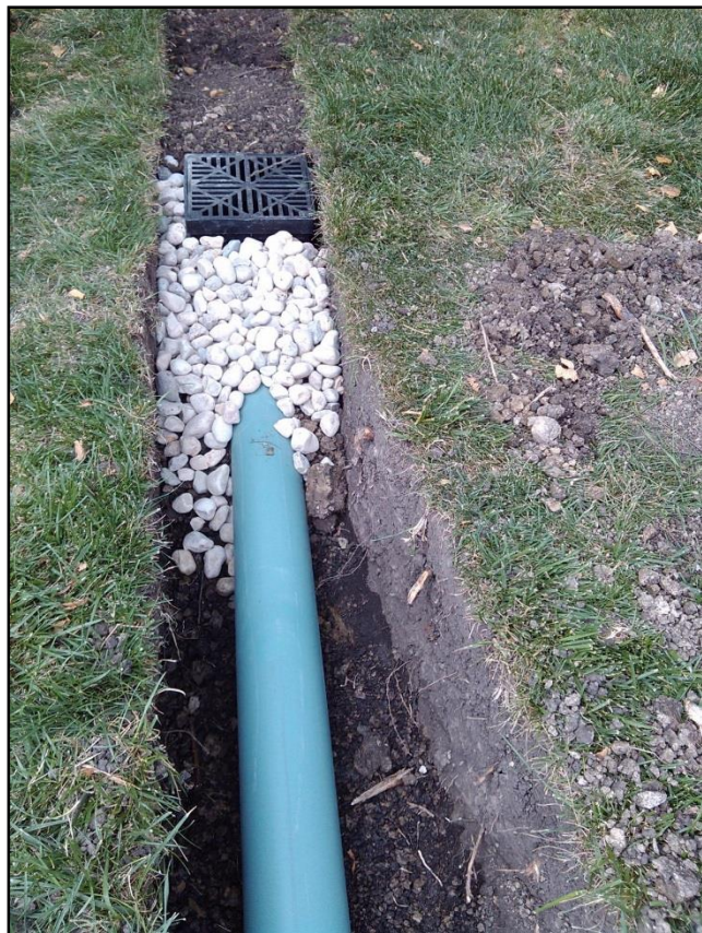
Photo 12 Solid PVC drainage pipe
