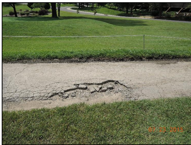
Photo 14 Deteriorating paths near 9 green
