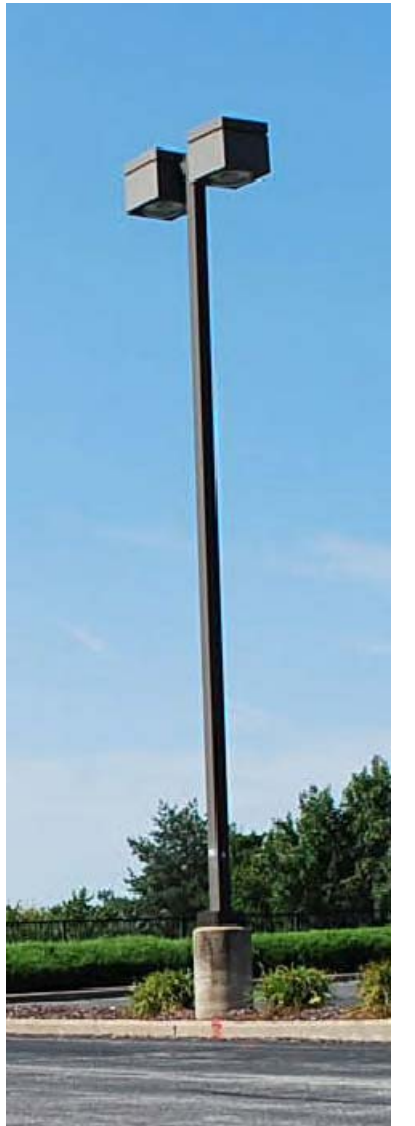
EXISTING SITE LIGHTING FIXTURES
