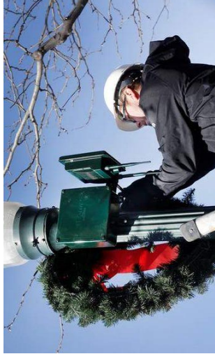
Retrofit for WIFI and other equipment
