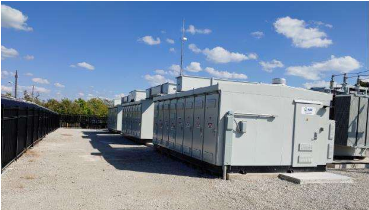
Figure 4: Applicants example photo of switchgear equipment
