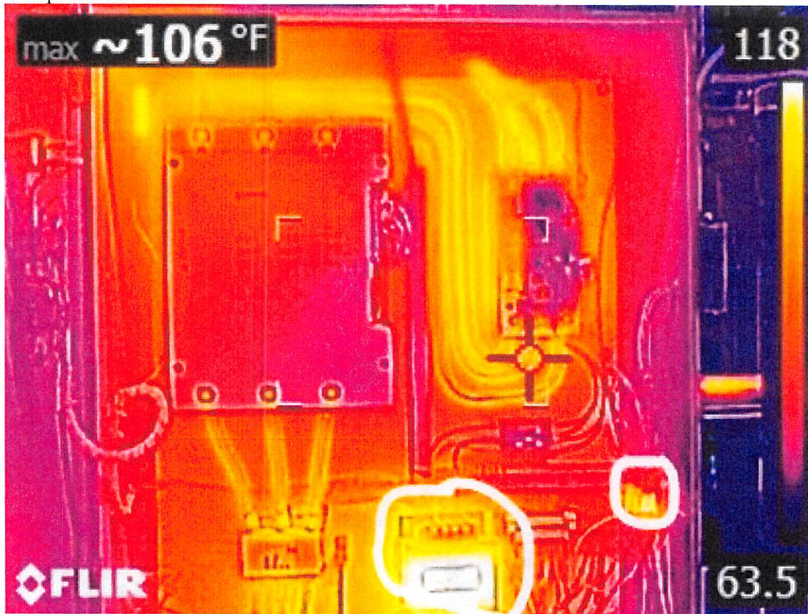
Compressor Two Panel
