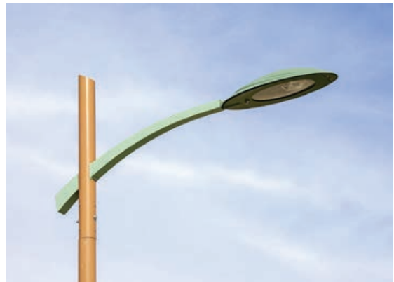
Parking lot lighting
