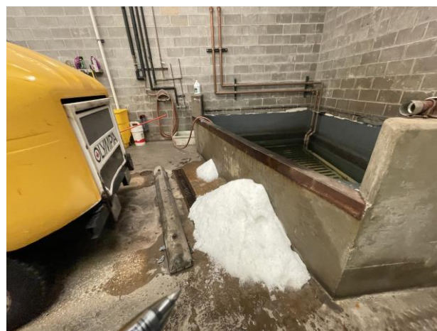
Photo 4 – Existing snow melt pit and coil
