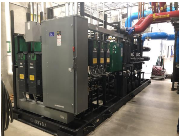
Photo 11 - Example of an Indirect CO 2 Chiller Package
