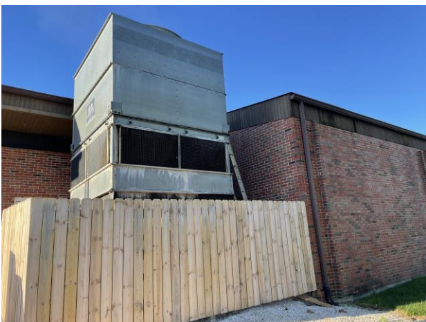
Photo 3 – Existing evaporative condenser
