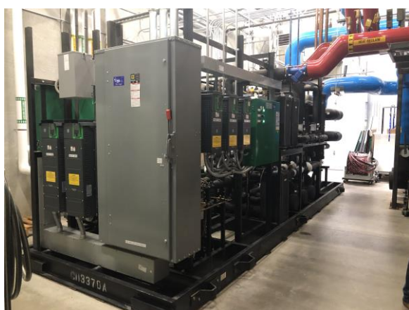
Photo 11 - Example of an Indirect CO 2 Chiller Package
