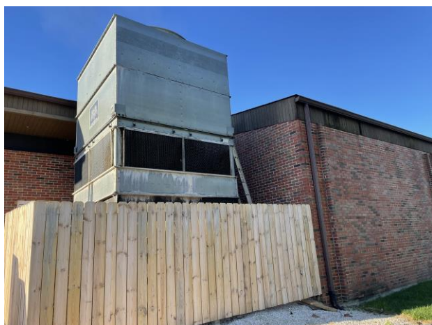
Photo 3 – Existing evaporative condenser
