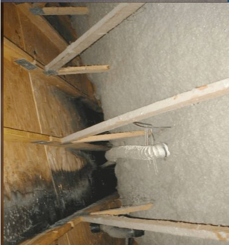
Mechanical System Defects
