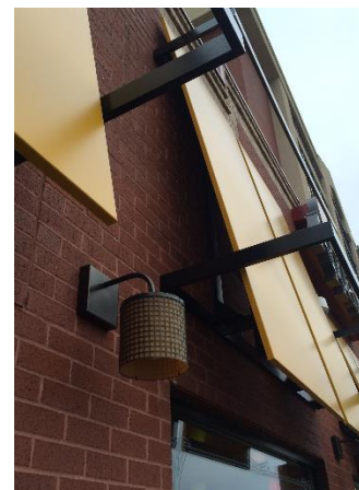
Figure 4: Close-up of new light fixtures
