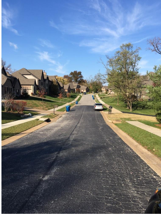
View of the existing conditions looking north from Ladue Road. City will contract to fill-in missing sidewalk sections, repairs to curbing and areas of sidewalk that have excessive cross slope.
