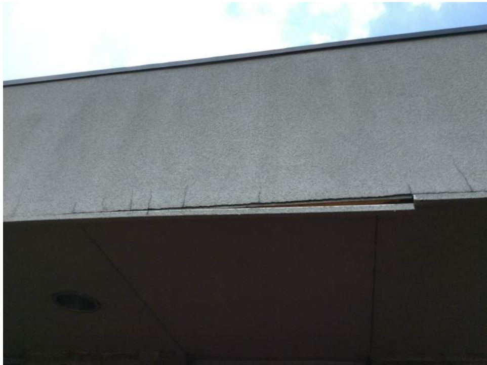
EXISTING CANOPY DAMAGE
