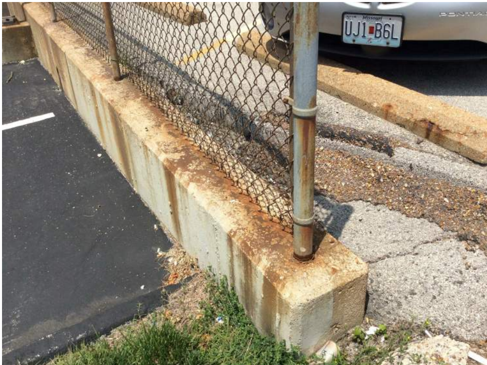
EXISTING RUSTING FENCE DETAIL
