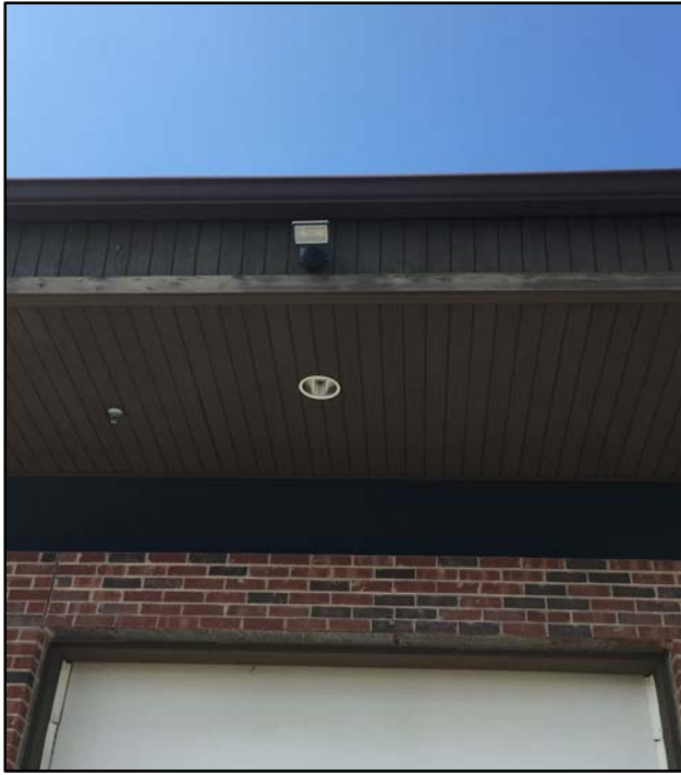
Figure 2. Existing wall-mount lighting and soffit lighting at the eastern Dielmann Recreation Complex parking lot.
