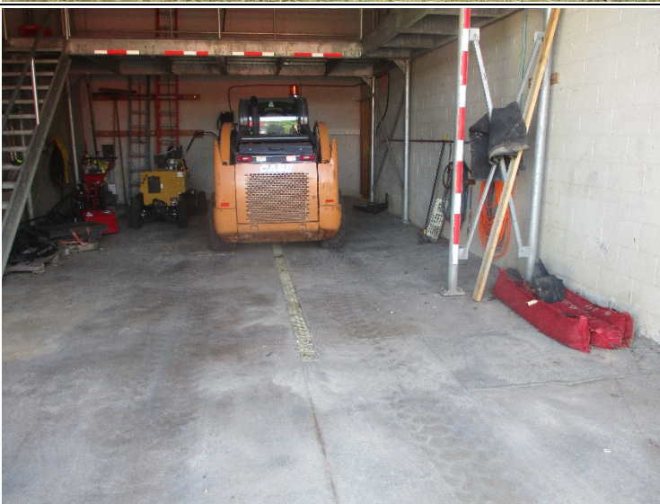
Photograph: #09 Taken By: Josh Rivers Date Taken: 8/17/2021 Program: WPC Unit Entity: City of Creve Coeur Permit: MOR040005 Location: Public works yard Description: Wash bay for city vehicles. Drain leads to oil water separator.
