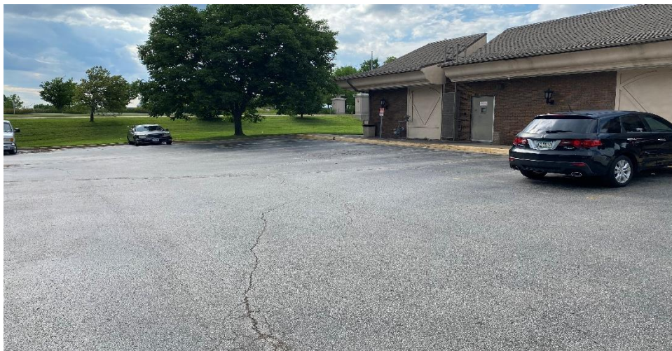
Figure 4: Lion's Choice parking lot with no visible parking space markings.
