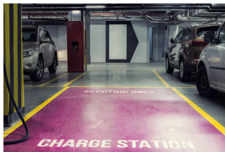
Multi-Family Dwelling Charging
