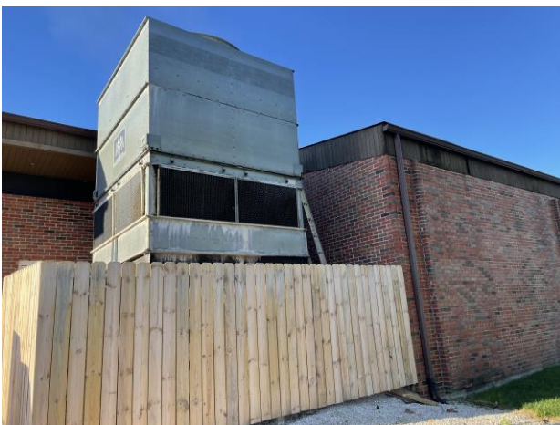
Photo 3 – Existing evaporative condenser
