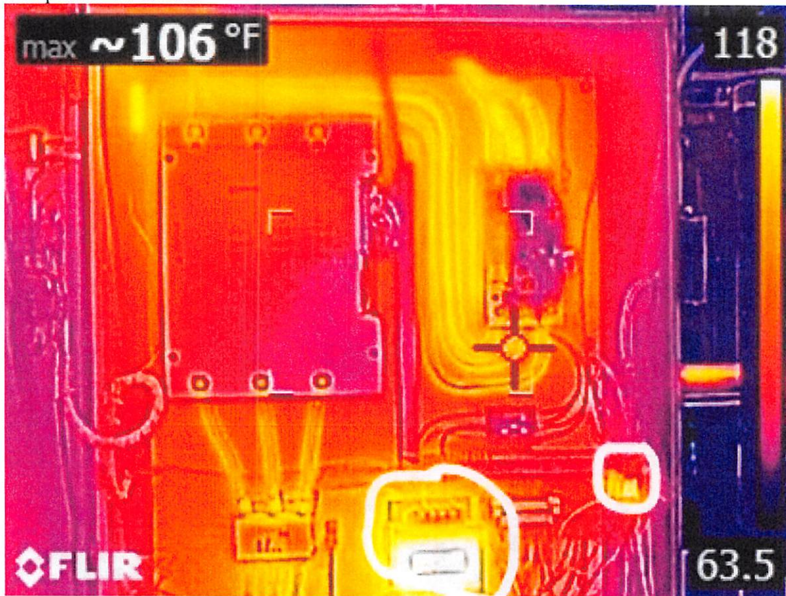
Compressor Two Panel
